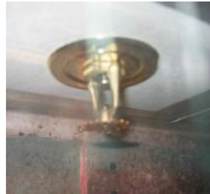
Pendent sprinkler after operation, viewed through window
