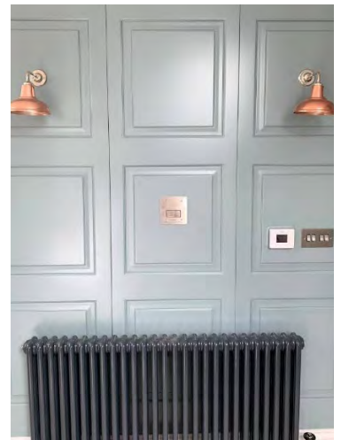
Figure 24: Above a radiator
