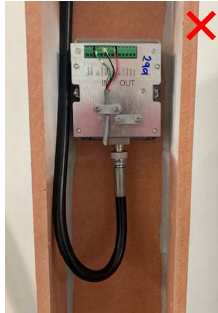
Figure 54: At risk trunking installation with hose bending
